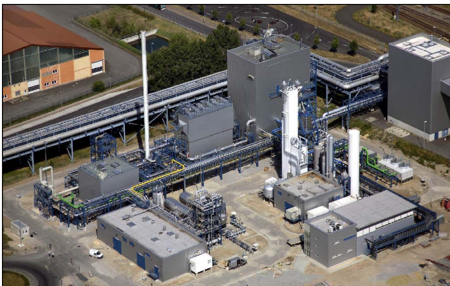
Figure 22. Oxy-Combustion Pilot Plant Capturing CO 2 from the Flue Gas of a Coal-Fired Boiler at the Schwarze Pumpe Power Station in Germany
